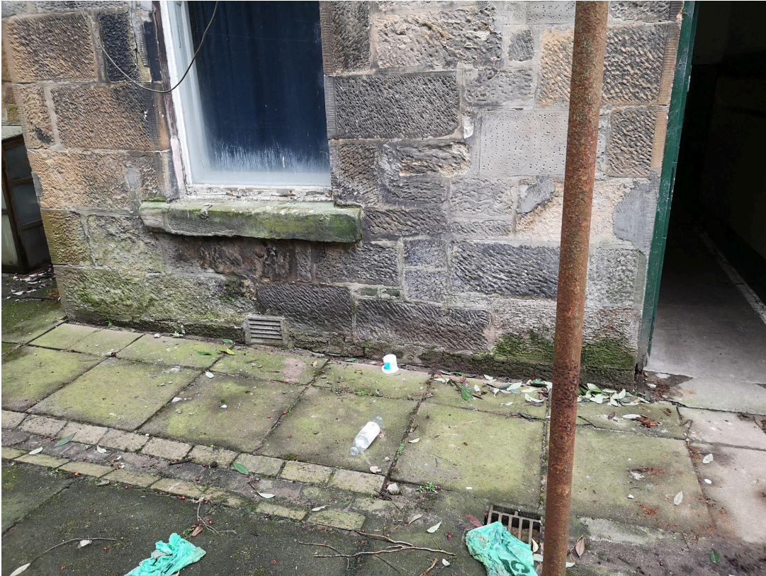
Figure 4.7: View of rear wall showing that the ground level is non porous and relatively high compared with floor joist position. There is some risk that floor joists may become wet and rot and this would be exacerbated by floor insulation. This risk is mitigated by the slope away from the wall towards a gutter and drain.
