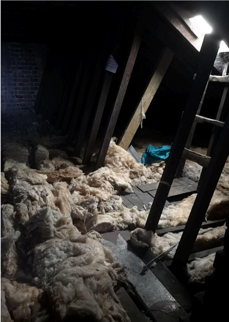
Figure 4.6: Incomplete 270mm insulation in the roof
