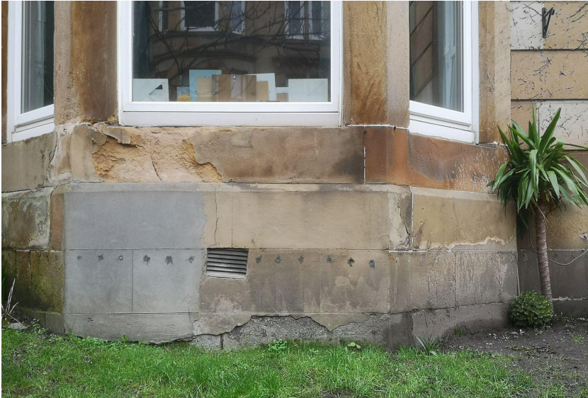
Figure 4.4: inappropriate cement repairs and ensuing surface delamination on the front wall.
