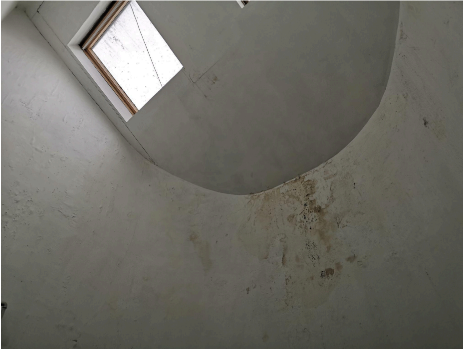
Figure 4.5: moisture damage in the stairwell at top floor.
